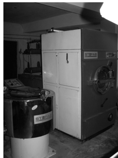
HYDRO EXTRACTOR & DRY-CLEANING PLANT
