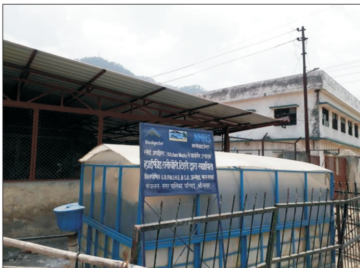
Biodigester Plant, Srinagar
