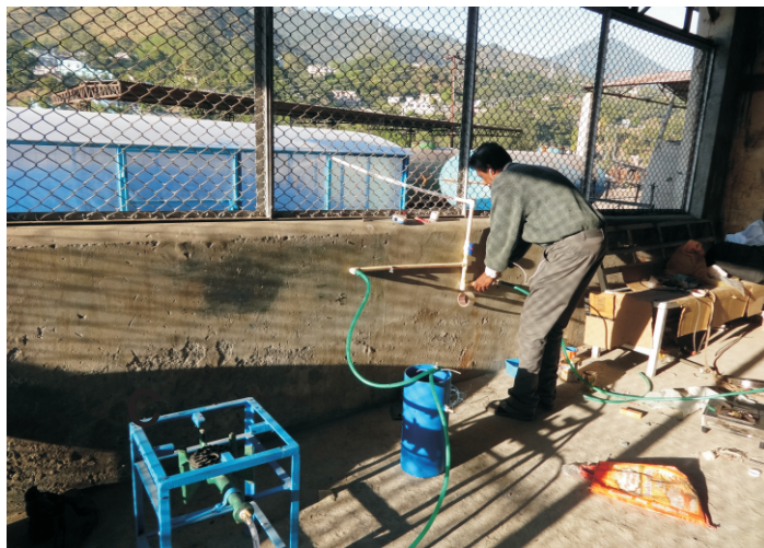
Biomethane, Biogas & Bioslurry Digester Plant, Srinagar
