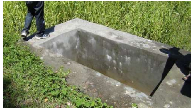
WATER TANK CONSTRUCTED UNDER THE PROJECT
