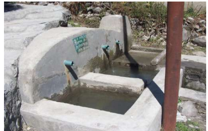
WATER TANK CONSTRUCTED UNDER THE PROJECT
