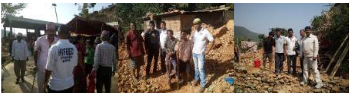
Reconstruction of Houses in Disaster Prone Area of Nepal by Hifeed Team
